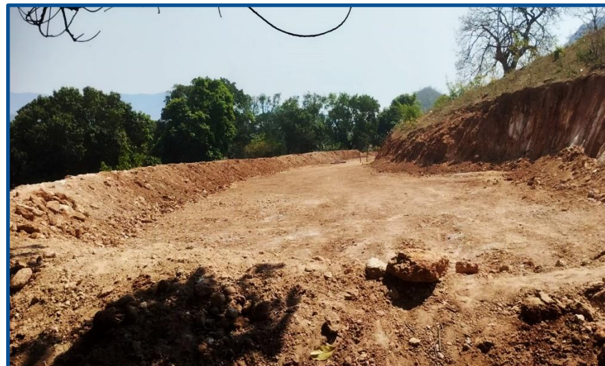
The rain water harvesting structure at Boripai (27 th March 2025), Rayagada district
